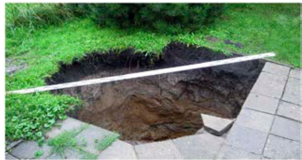
Figure 4. Sinkhole created inside the area of the building plot over the old shallow mining workings
