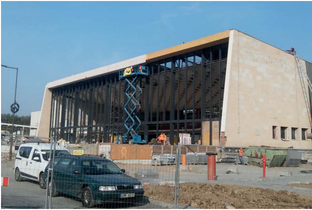
Ill. 12. Remodeling — non-proportional thickness of the roof face (2020).
