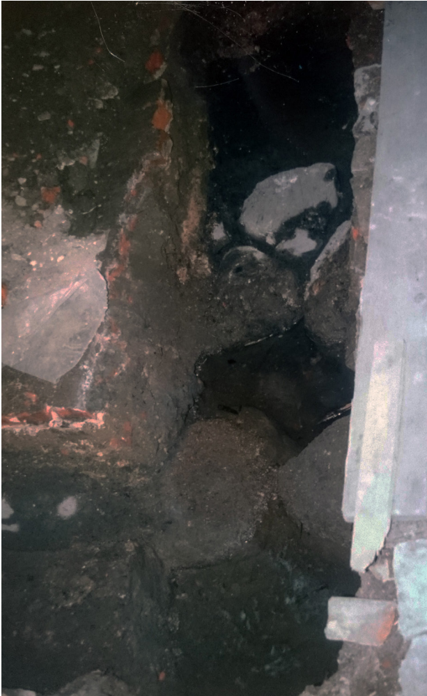
Fig. 5. Relics of the lowest parts of the foundations discovered during the 2003 excavations (photo by D. Biernat [12])
