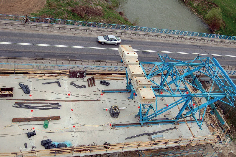
Fig. 5. Exemplary arrangement of temporary benchmarks (points in red) on the span deck of the structure in Łabuzie
