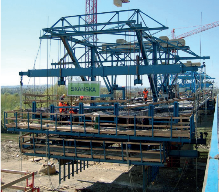
Fig. 3. View of the girder and the scaffolding trolley at the construction site of the bridge in Łabuzie
