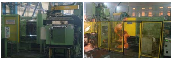
Fig. 2 Production machine for Workstation L20-630.05
