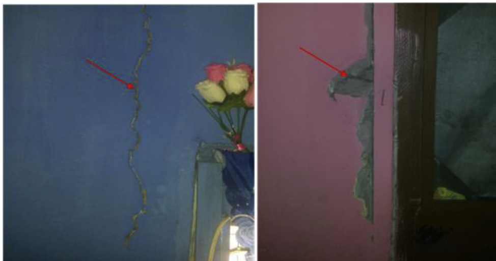
Fig. 3 – Cracks in the walls (bedrooms) of Building Structures at Nkanponase. Residents attribute the cracks to blasting activities by small scale miners.
