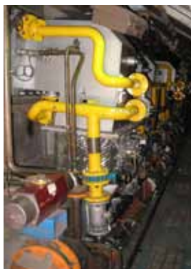
Fig. 1. Photo of the HTB burner
