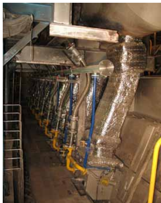
Fig. 6. Photo of the HTB burners, zone 3, SSAB
