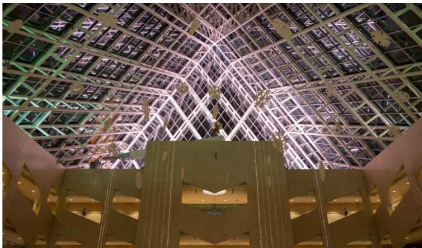
Fig. 3. Roof structure of Edmonton City Hall, Edmonton, Canada (author of photography: Mack Male [10])
