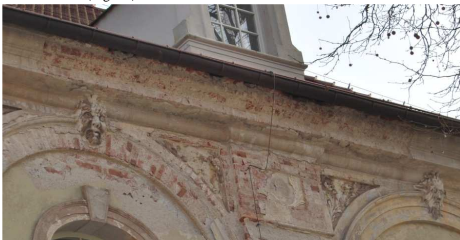
Fig. 10. Deteriorating east façade (fot. W. Sokołowski)
