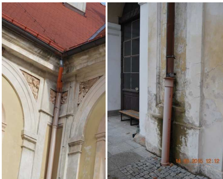
Fig. 12, 13. Existing connections of the downspouts on the east façade (fot. W. Sokołowski)
