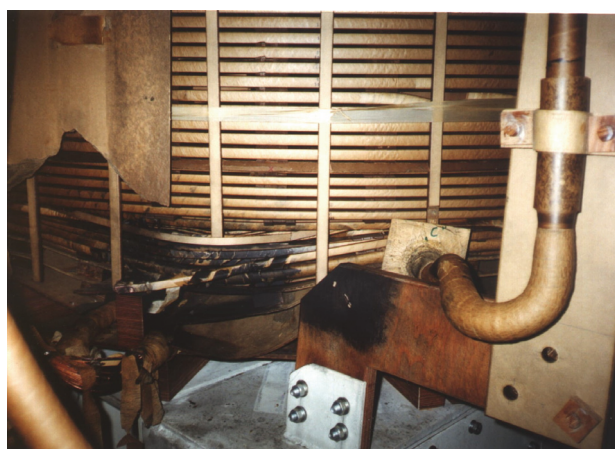
Fig. 4. Deformation of the lower part of the HV winding of the analysed autotransformer
