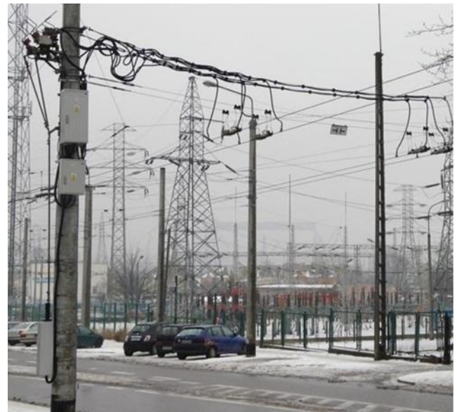
Fig. 6: Remotely controlled disconnectors of the overhead line (the city of Gdynia).
