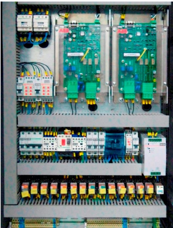
Fig. 13. Interior of the field circuits power supply cubicle with the FEX4 boards
