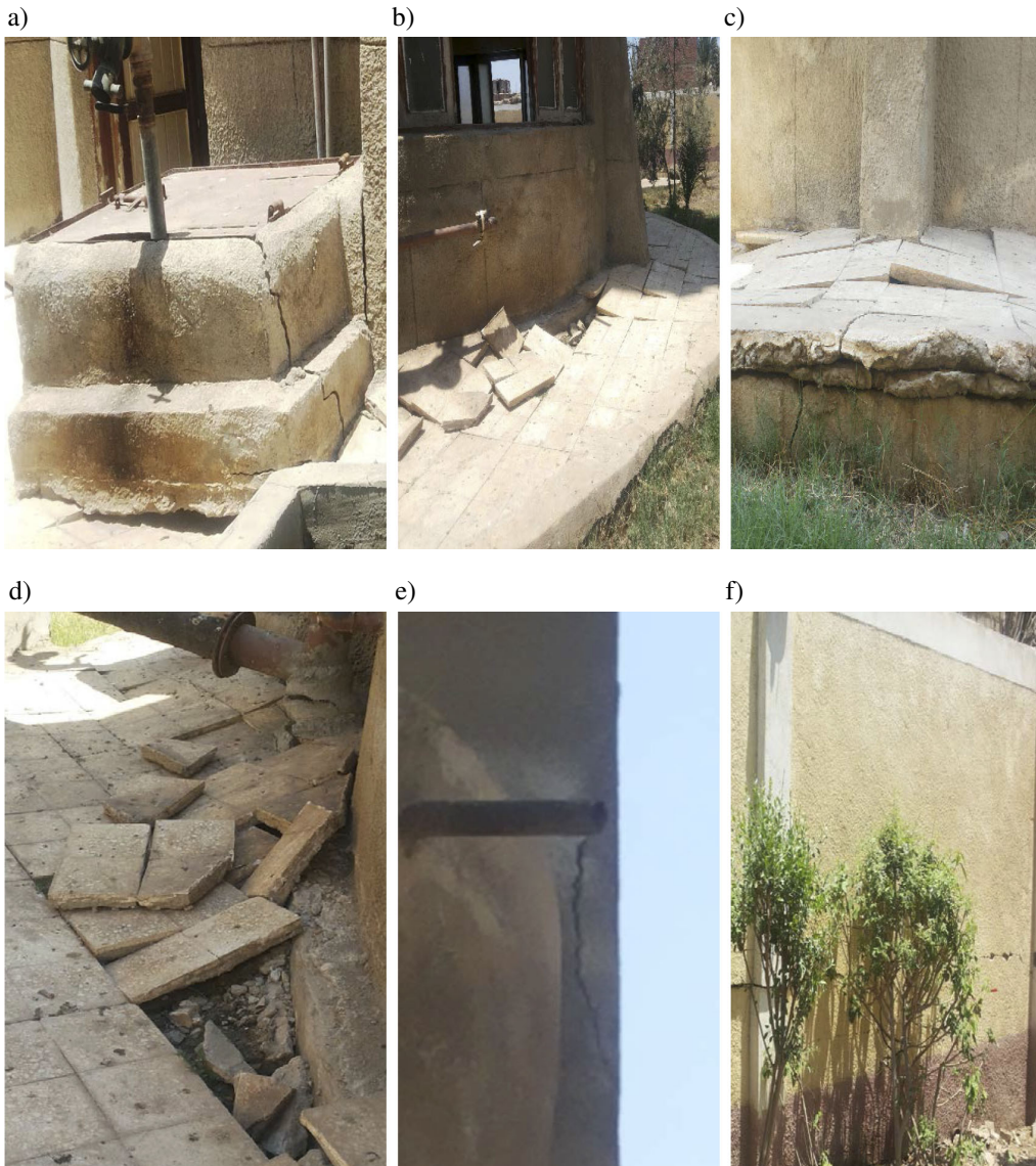
Fig. 3. Cracks in the water storage tank and surrounding wall (July 2014). a) Cracks near a pump; b) Cracks in the base of the tank; c) Cracks in base of the tank; d) Cracks in the base near the skeleton; e) Cracks in the concrete structure; f) Cracks in a common brick wall
