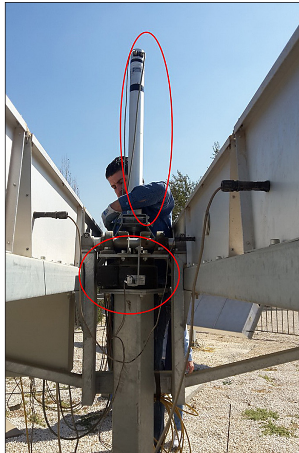
Figure 13. Both motors for CPV system
