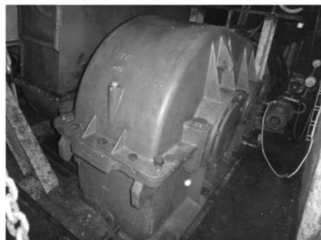
Fig. 1. Flender multi-stage angular-cylindrical gear unit with visible circulating lubrication system
