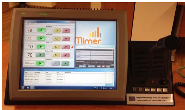
Figure 6. VHF operator workstation at the RIS-PL Operating Centre.
