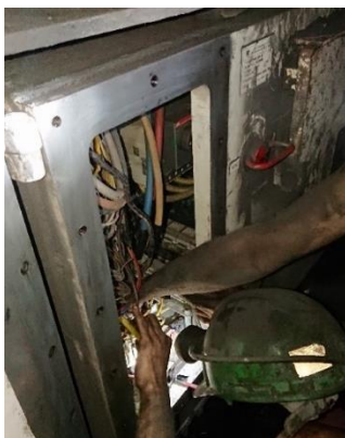
Fig. 4 Repair of apparatus box failures
