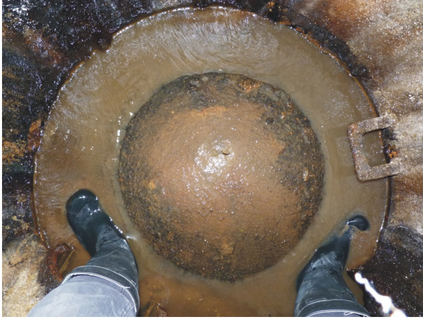
Fig. 5. A bulge caused by groundwater pressure in geotextile at the bottom of a well
