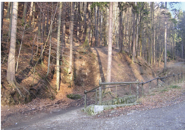
Fig. 5. Drift sinkhole within the boundaries of archeological site Lubachów 2 (AZP 87-23) (photo by T. Stolarczyk)
