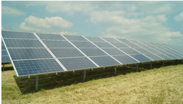
Fig. 1. Photovoltaic power plant in eastern Poland
