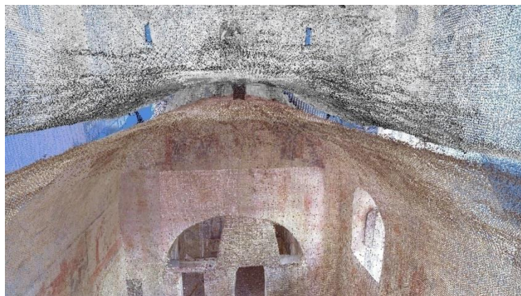
Figure 9. Detail of the vault of the nave, obtained with the ReCap software
