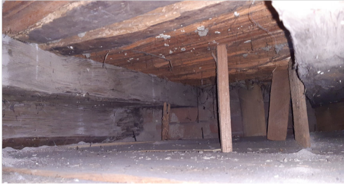
Fig. 7. View of the ceiling cross-section taken with an endoscopic camera
