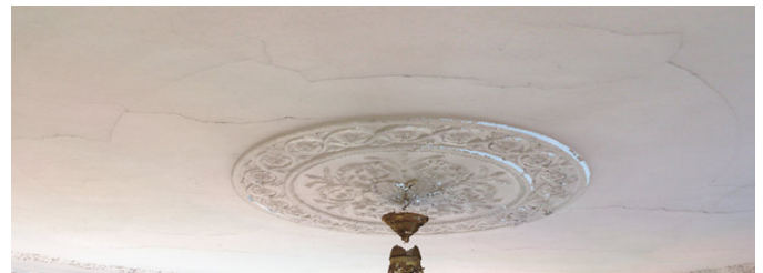
Fig. 6. Stucco on the ceiling (visible cracks in the plaster)
