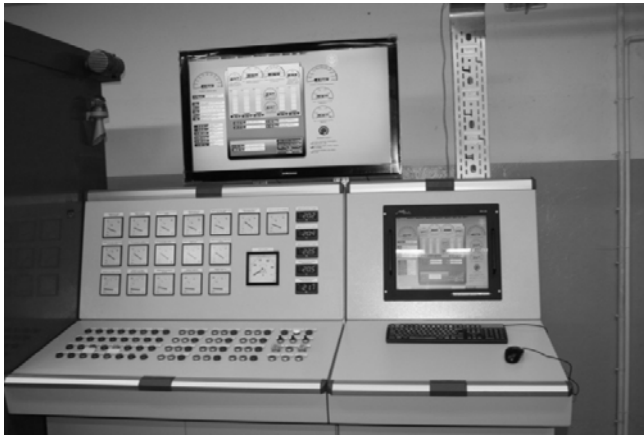
Figure 2. Operator station EMOS
