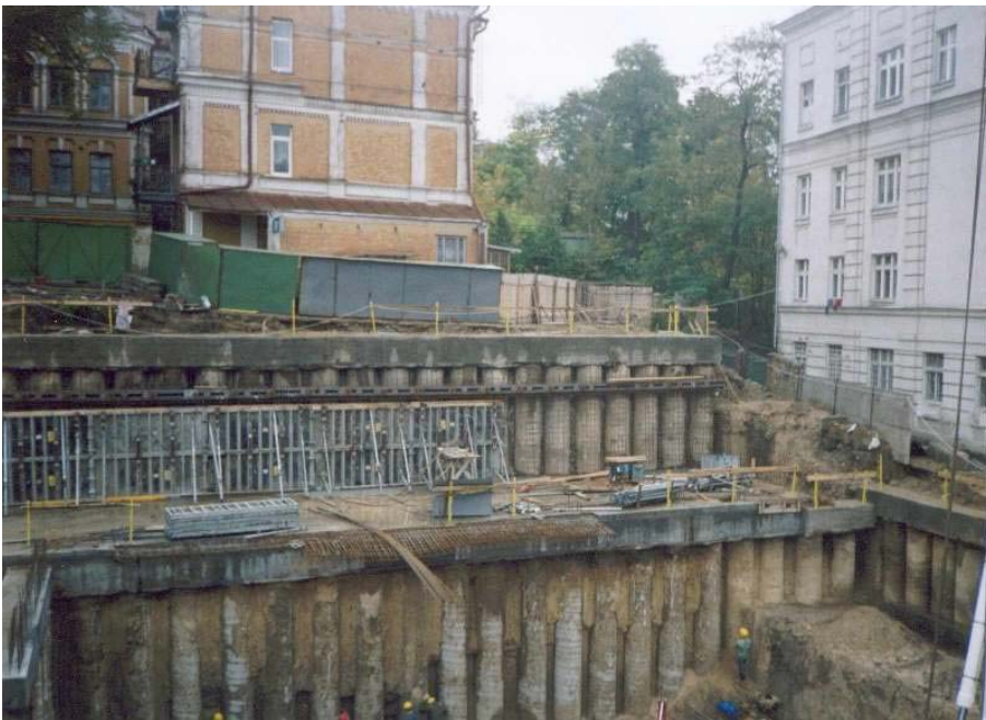
Fig.4. An example of the deep excavation for the new construction in the conditions of dense buildings and complex geological conditions in the Pechersk district of the Kyiv city. Source: the author's photo
