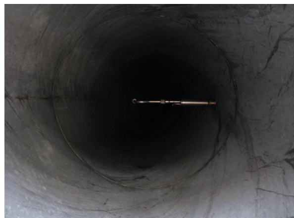
Fig. 2b. Measuring probe with the filter installed in the tested ventube pipeline
