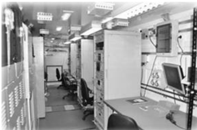
Fig. 7. Mobile Metrological Laboratory inside view
