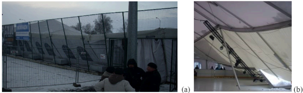
Fig. 3. Disaster of tent hall laden with snow a) external view, b) damaged aluminum girders of ice rink roof in Szczecin, photo PINB Szczecin (public domain) [45]
