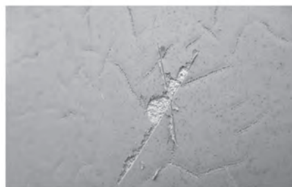
Fig. 8. Examples of measurement locations in the damage area
