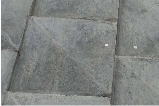
Fig. 8. Reflective tape targets on reinforced concrete facing on the opposite sides of the expansion joint
