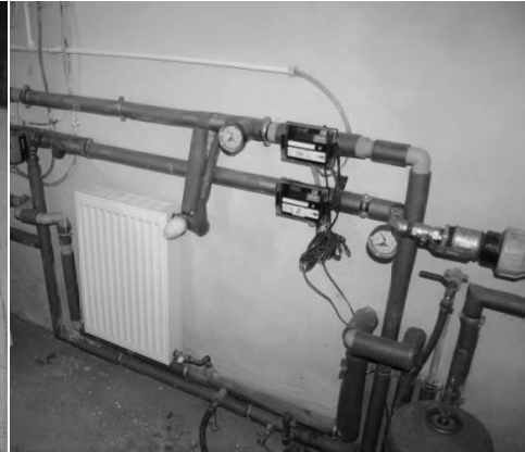
Figure 4. Installation with heat meters
