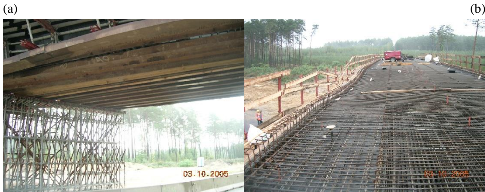
Fig. 5. View of viaduct WD-12 scaffold after vehicle strike: (a) damaged and turned steel girders of scaffold (two girders on Wrocław side were turned), (b) collapsed reinforcement of span load-bearing structure before planned casting.
