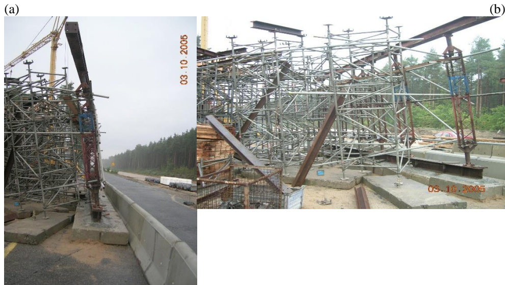
Fig. 4. View on the damaged scaffold supports in viaduct WD-14 after vehicle struck to the main girders located above drive-through clearance: (a) view from roadway, (b) side view.
