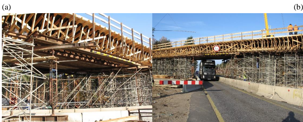
Fig. 6. Side view of encased scaffold of viaduct WD-14 prior to superstructure casting after two vehicle strikes into girders located above clearance: a) H20 scaffolds erected under formwork, b) drive-through clearance outline shifted to edge of roadway.
