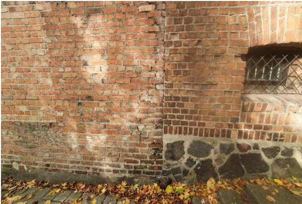
Photo. 2: No masonry bond at the junction of the former office spaces (A) with the former staff apartment (B), part of which are the rooms of the Southern Guardhouse
