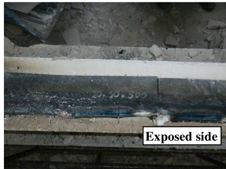
Linear joint seal No. II extent of thermal degradation – 21,8 mm
