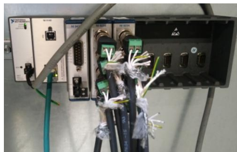
Fig. 10b. Additional chassis for accelerometers connection
