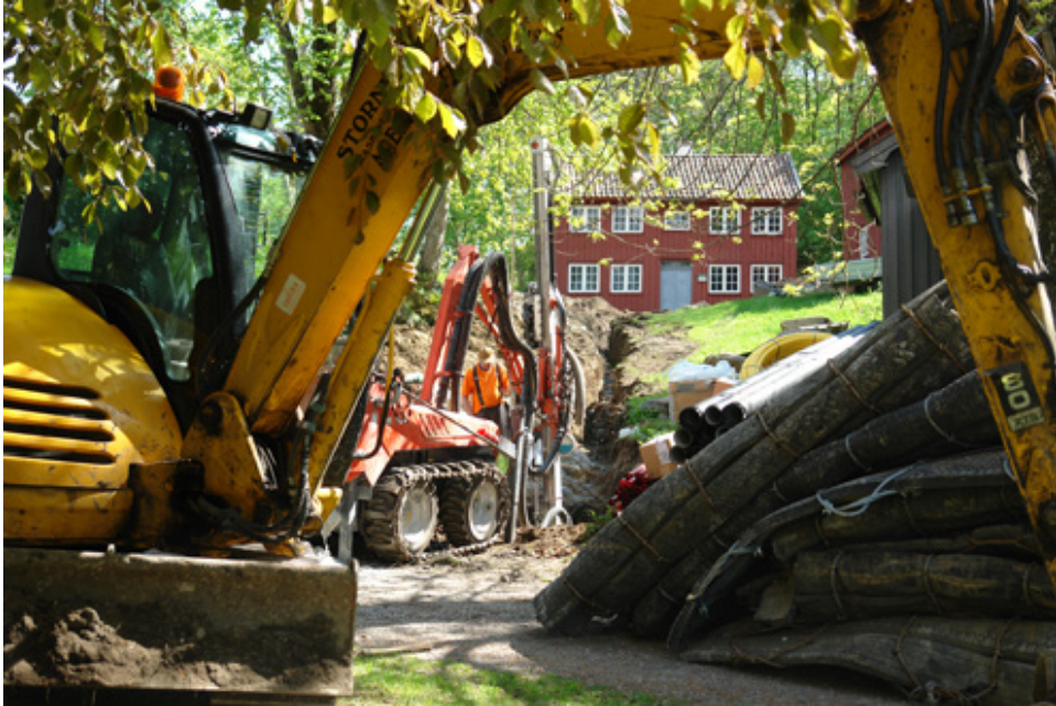
Fig. 5 The restoration of Enghavehuset required a project group consisting of eight different professions, with everything from conservator to demolition expert. All in all, this little house had apx. 15 people working on different aspects of the restoration during the project. Photo: Tanja Røskar
