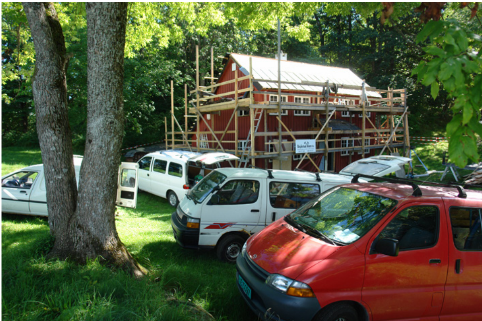
Fig. 6 On any given day there could be 4-5 different types of craftspeople present on-site. This resulted in a parking problem that was larger than any cooperation problems. Photo: Tanja Røskar
