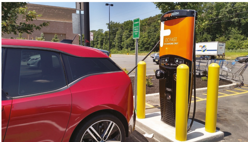
Fig. 1. Electric vehicles charging station
