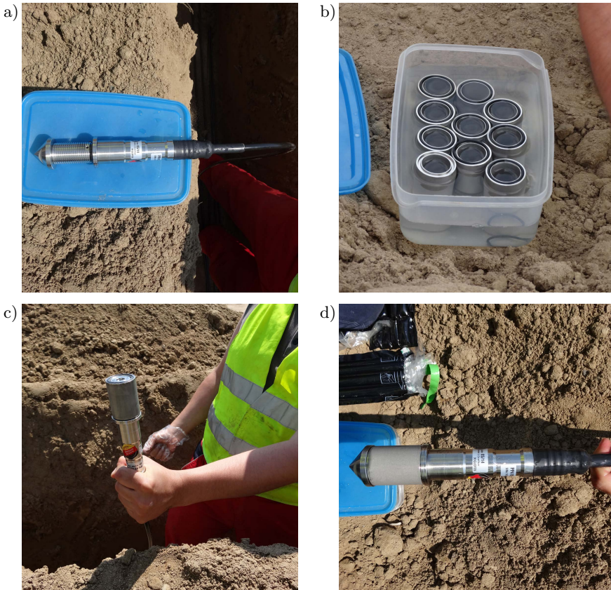
Figure 3. Installation of porometer: a) sensor prior to the installation of the filter, b) filters prior to the installation, c) filter installation, d) sensors after the installation of the filter [4].
