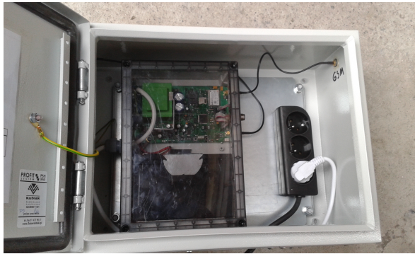
Figure 19. Edge Node with emergency power supply.
