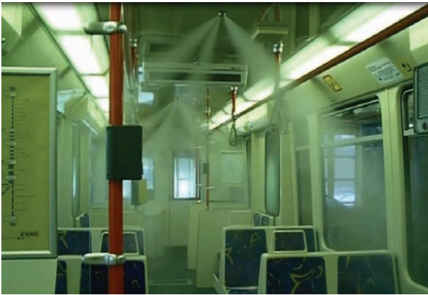
Fig. 2. High pressure water mist spraying in passenger train [16]
