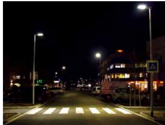
Fig.9. „Futurlux cross-walk” lighting system.
