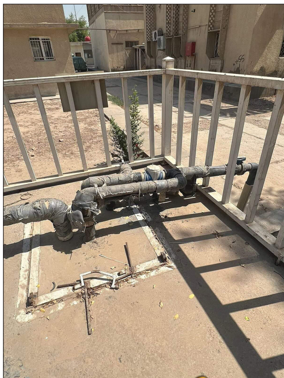
Figure 1. Discharging and transition pipe on top of the storage and decay system
