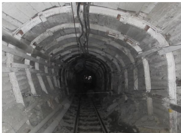
Fig. 2. Failure condition of the main haulage roadway
