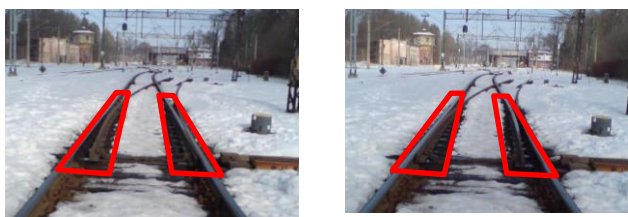
Fig. 1. Switch-point saver heating work area, for right and left point
