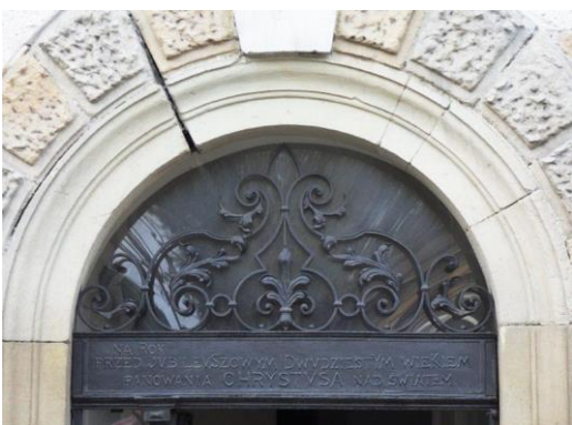
Fig. 8. Ironwork gate to the house Ekielski, and an inscription. Source: A. Jurek
