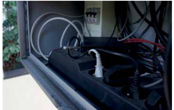
Fig. 4. Example of connecting GSM modem and other devices in a variable message sign to a power strip for domestic use [own study]
