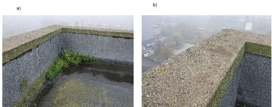
Figure 2. Grain Elevator building - roof level: decapitalization of: a) roofing felt (blistering and unevenness), b) cornice elements (carbonation)
