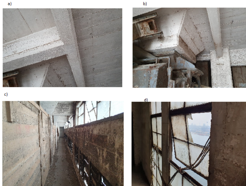
Figure 5. Grain Elevator building - level +5: a) mechanical damage to structural elements, b) equipment for transporting loose materials left inoperative and incomplete, decapitalization of: c) ventilation shutters, d) window joinery
