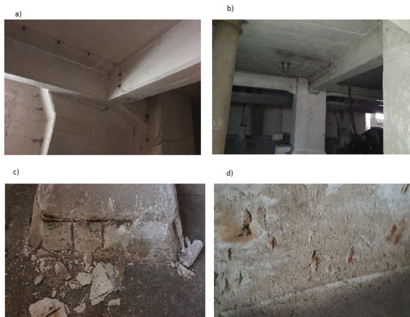
Figure 6. Grain Elevator building - level -1: a) mechanical damage to structural elements, floor zone: c) concrete cover falls off the column heads at the level of the foundation slab, d) moisture in the outer wall
