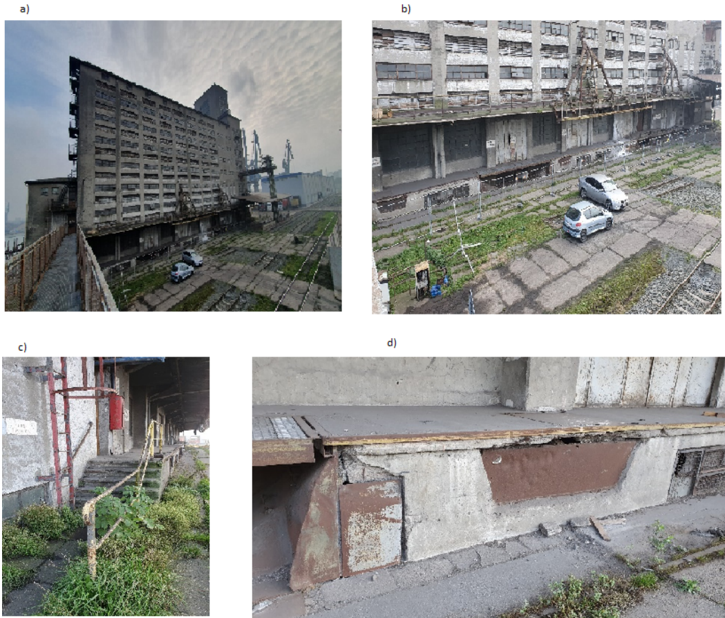
Figure 1. Grain Elevator building - elevation from the land side: a) general view, b) close-up, unloading ramp at the ground floor level: c) general view, d) damage in close-up
