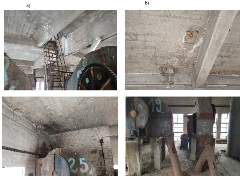
Figure 3. Grain Elevator building - level +10: a) mechanical damage to structural elements, b) defective and incomplete equipment for transporting loose materials
