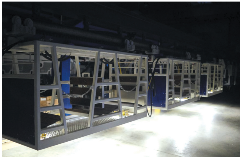
Fig. 4. Mobile lighting of passenger stations from the CA-190 battery-powered suspended locomotive (white light – the locomotive is at the passenger station)
