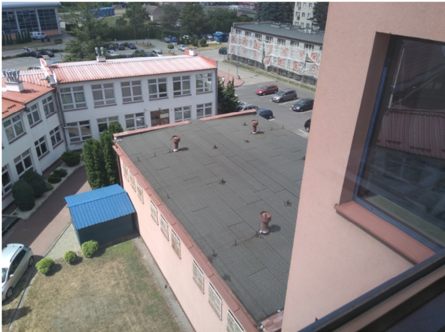
Fig. 1. Photography of the gym's flat roof, that is adjacent to P building at Rzeszów University of Technology
