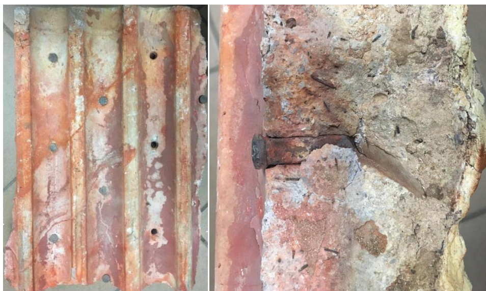
Fig. 1. Damaged ceramic refractory with visible anchors
