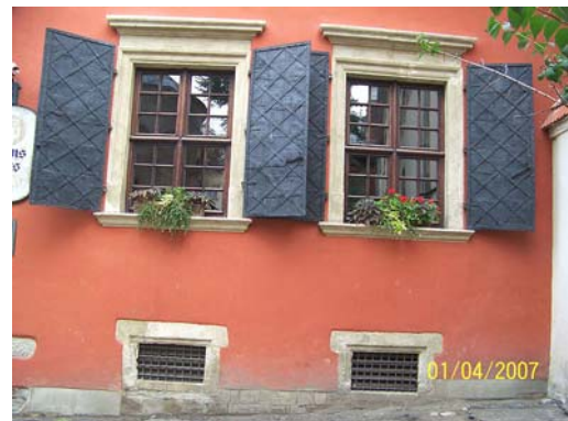
Fig. 9. The restoration of red façade surface and iron shutters of Armenian Lombard. Source: photo by author
