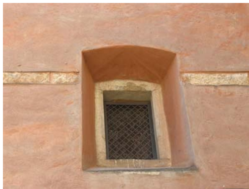
Fig. 8. The restoration of the polychromy of the façade surface and stone details of City Arsenal. Source: photo by author
