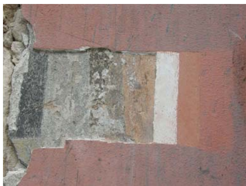
Fig. 4. Sounding of painting layers of the façade in 28, Market Square. The red color appears only in the 20 th century. Source: photo by author
