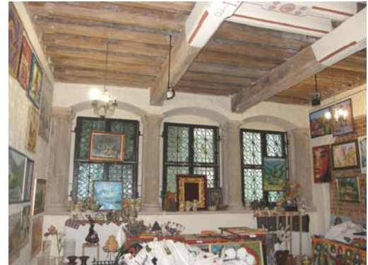
Fig. 14. The modern destruction of restored polychromy (the first floor, 37, Market Square). Source: photo by author
