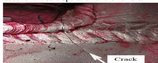
Fig.7. Cracks on a bolster beam of a Metro system
